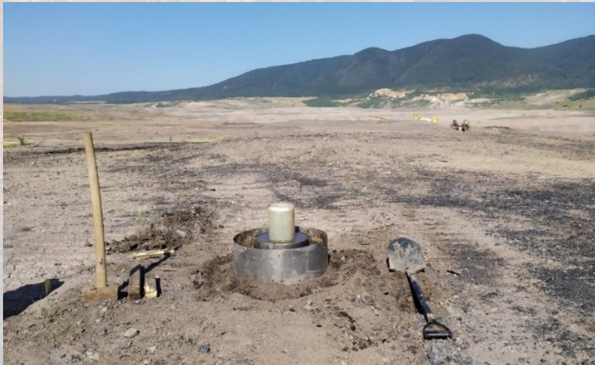
Figure 19 Procedure for carrying out infiltration tests on the internal wastedump of the ČSA mine.
